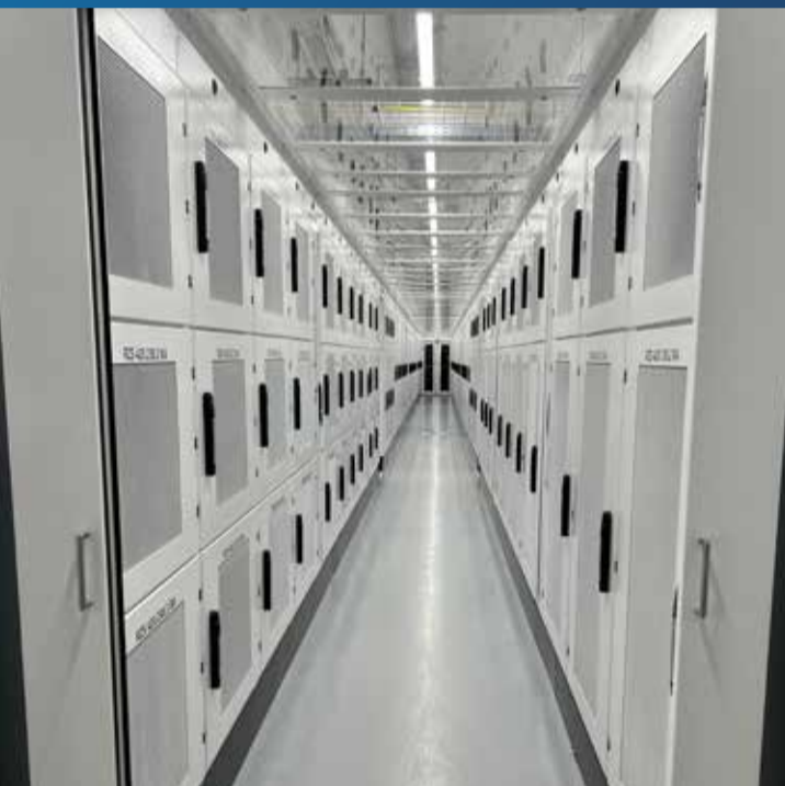
In the main and secondary tunnels, the cabinets with "Agent E Wireless" technology are installed in cold aisle enclosures.
